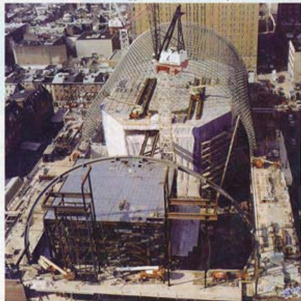
MANY FACETS Steel erector used hall roofs to access vault. Arch is built on bents.
